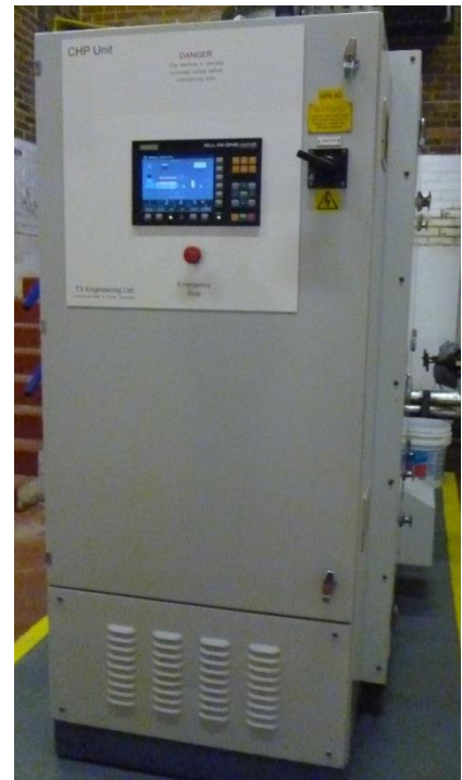
CHP unit at Dewsbury Sports Centre
