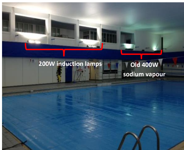
The Pool hall at Batley Sports and Tennis Centre. Left: 200kW induction lamps (natural daylight colour, with good light dispersion). Right: Old 400kW lamps (tinted colour, poorer light dispersion).
